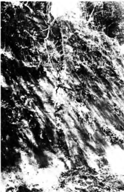
Photo : Cracks developed on the cladding wall with lateral shifting.
