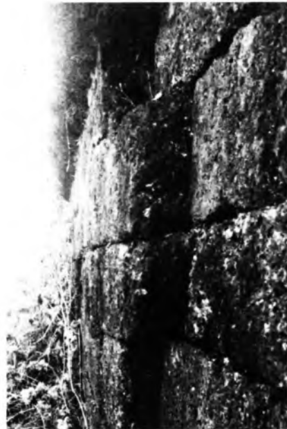
Photo : Old sea wall showing lateral shifting along the vertical cracks
